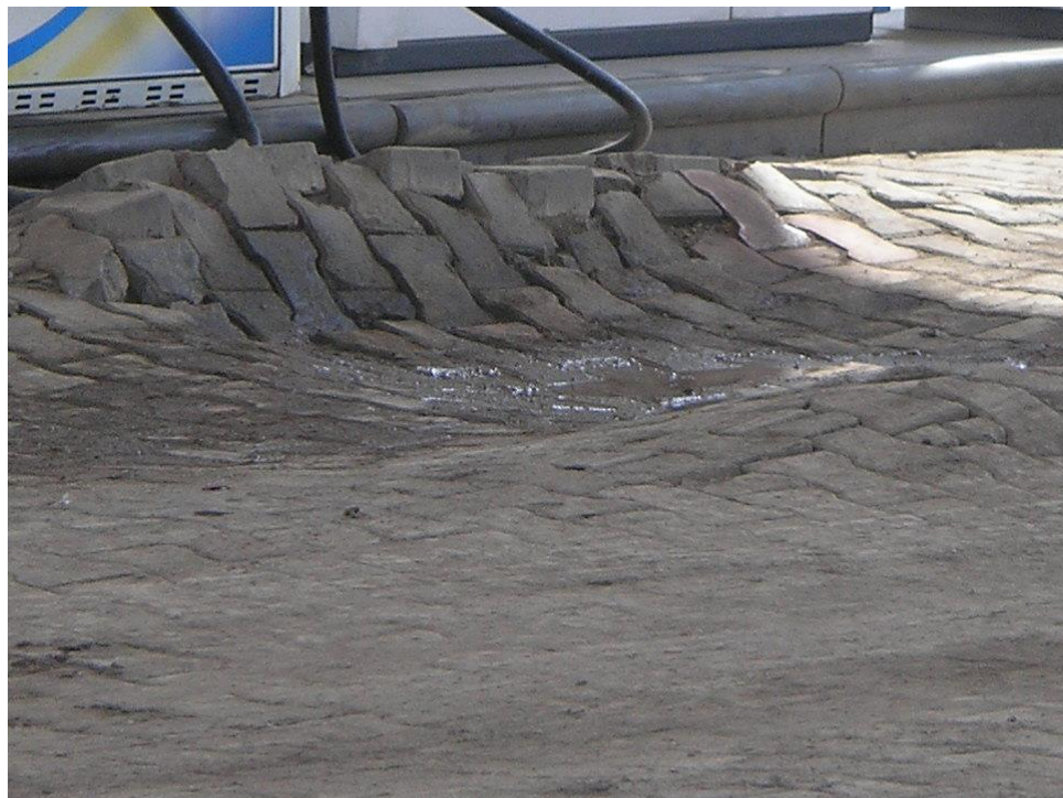
Fig. 16 Forensic GT Investigation of Distress of floor of a Petroleum Retail Outlet
