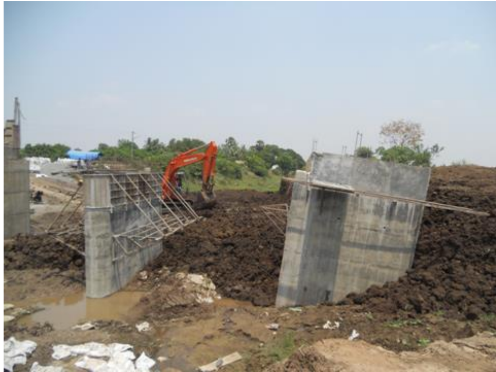
Fig. 15 Forensic Geotechnical Investigation of tilt of a Bridge abutment
